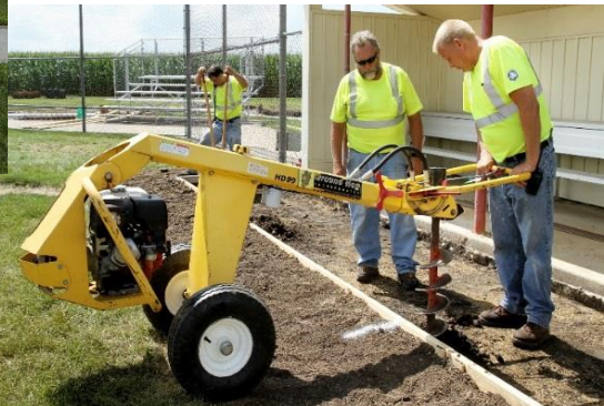
Baseball/Softball dugout project
