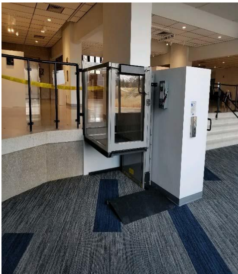
Patio Entrance Wheelchair Lift
