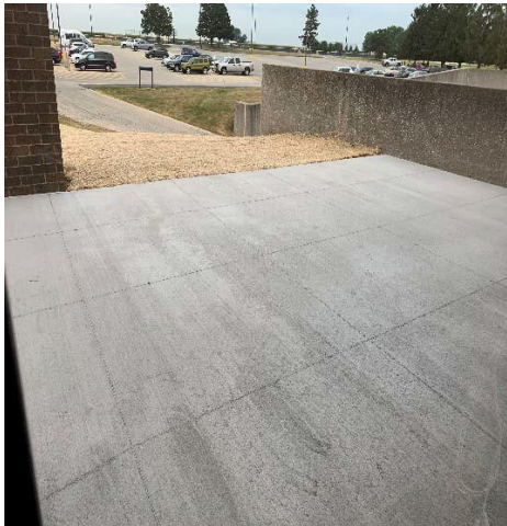
PHS – Emergency Library Ramp
