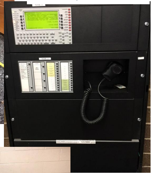
The Main Campus - PHS Fire Alarm
